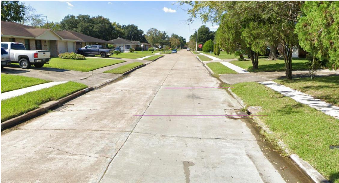
Knotty Oaks Trail- Substandard inlets
